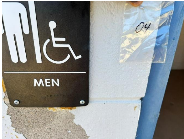
2. Sample #04 – door caulking
